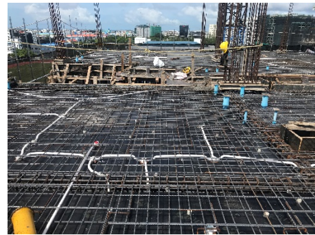
9th Floor Plumbing & Electrical Sleeve
