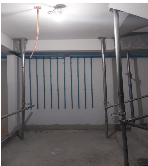
10 th floor fresh water line
