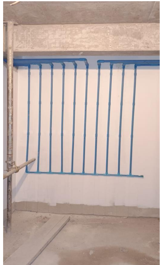
3 rd floor fresh water line
