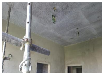
5 th floor type C wiring
