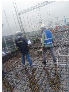
13th Floor Electrical & Plumbing Sleeve
