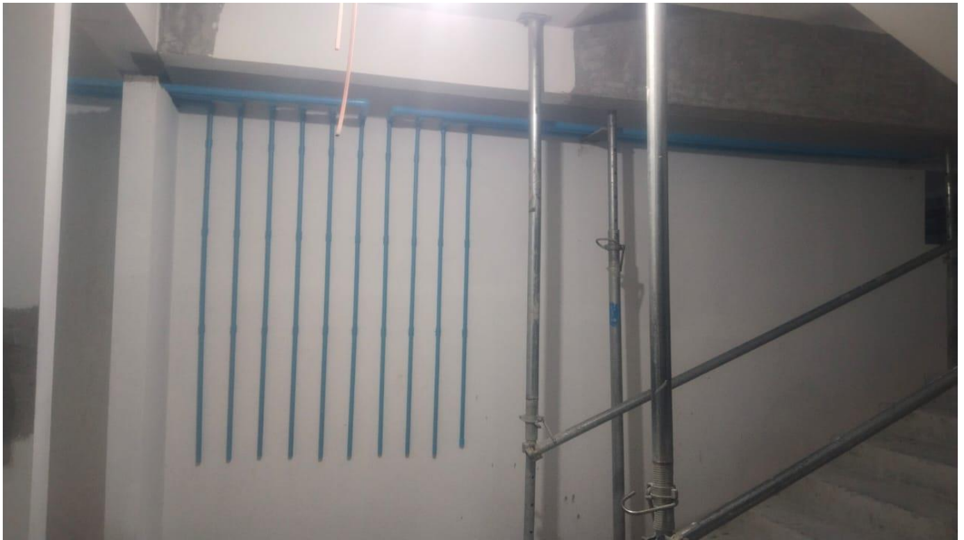
12 th floor fresh water line
