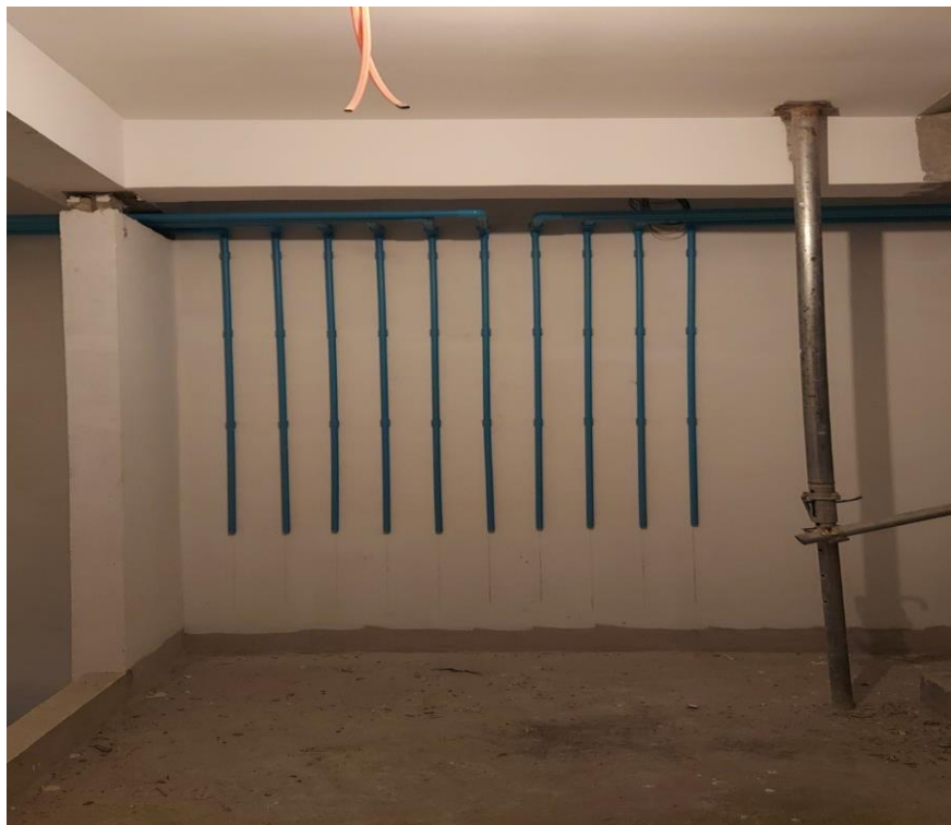
5 th floor fresh water line
